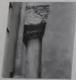
Fig. 214. S. Susanna. Wall of south aisle, showing column and spring of arch.
